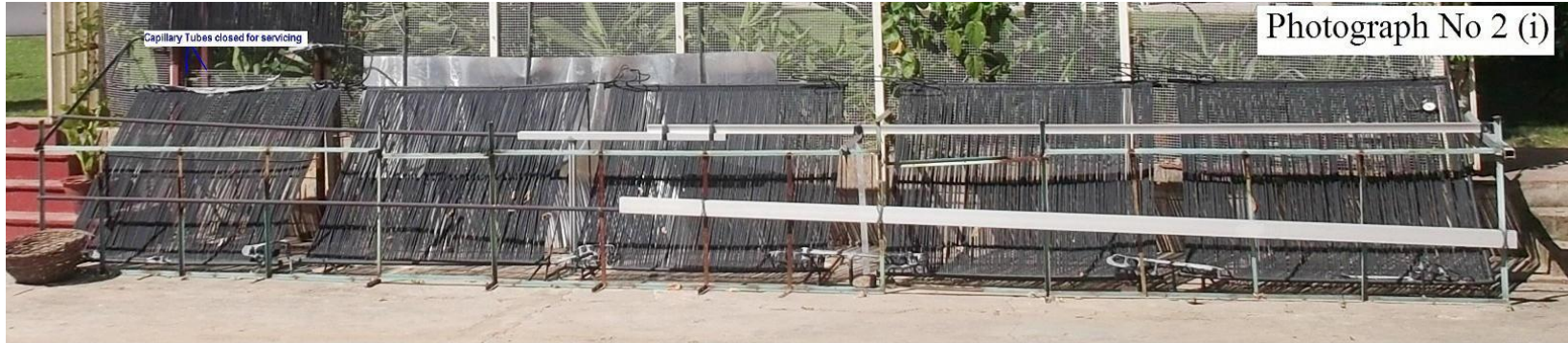
Heating Assembly – 5 Heating Assembly units , No's 1,2,3,4 & 5 inter-connected to each other .
