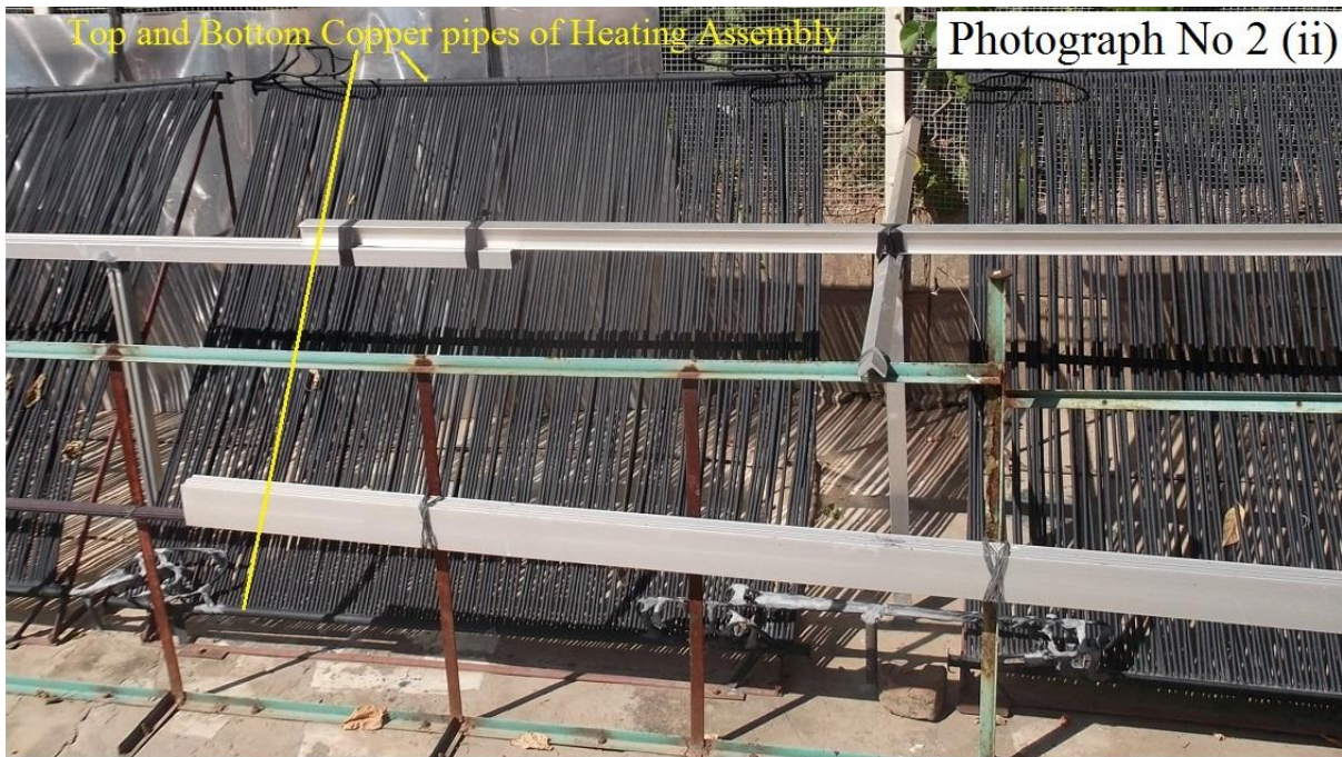
Assembly of 5 Heating Units Inter-Connected to each other, both at the top (for Vapour flow) and at the bottom (for Liquid Diethyl ether flow)
