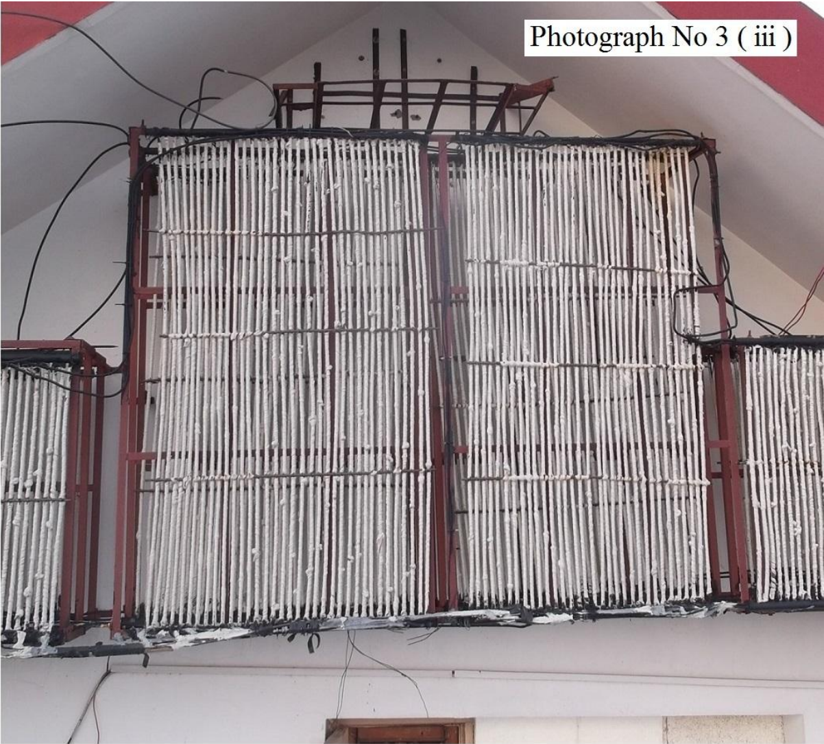
Close-up view of the Cooling Assembly
