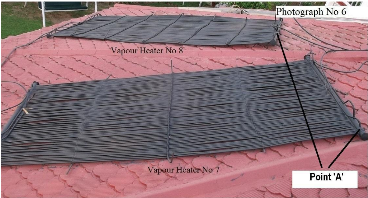
Vapour Heater No. 7 and No. 8
